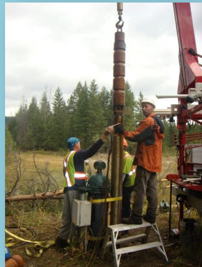
New Well Pump
