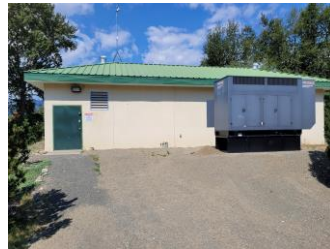
Community Water Backup Generator
