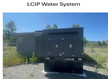
LCIP Water System
