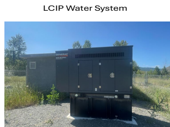
LCIP Water System
