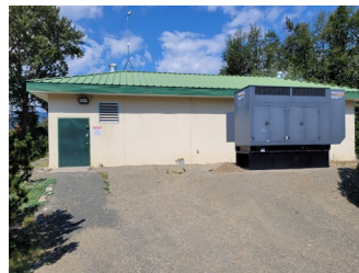
Community Water Backup Generator
