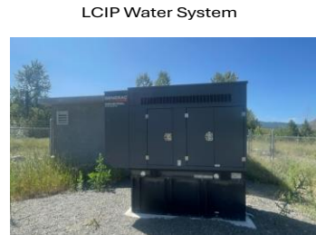
LCIP Water System
