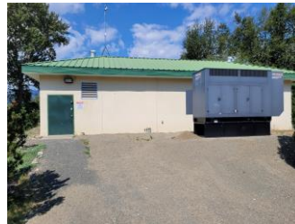
Community Water Backup Generator
