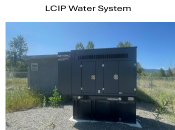
LCIP Water System
